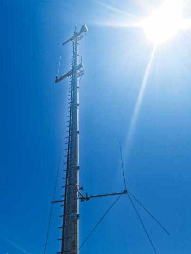
Figure 3 CEO Substation at the Aguçadoura Test Site – tower to support communications and surveillance. (Photo credits: INESC TEC)
