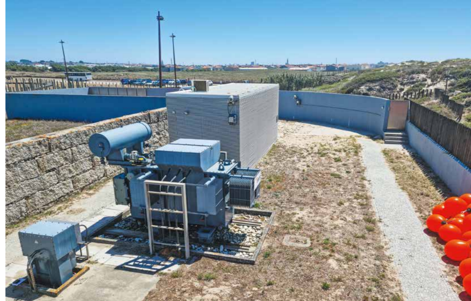
Figure 4 CEO Substation at the Aguçadoura Test Site - transformer and the subsea cable connection point. (Photo credits: INESC TEC)
