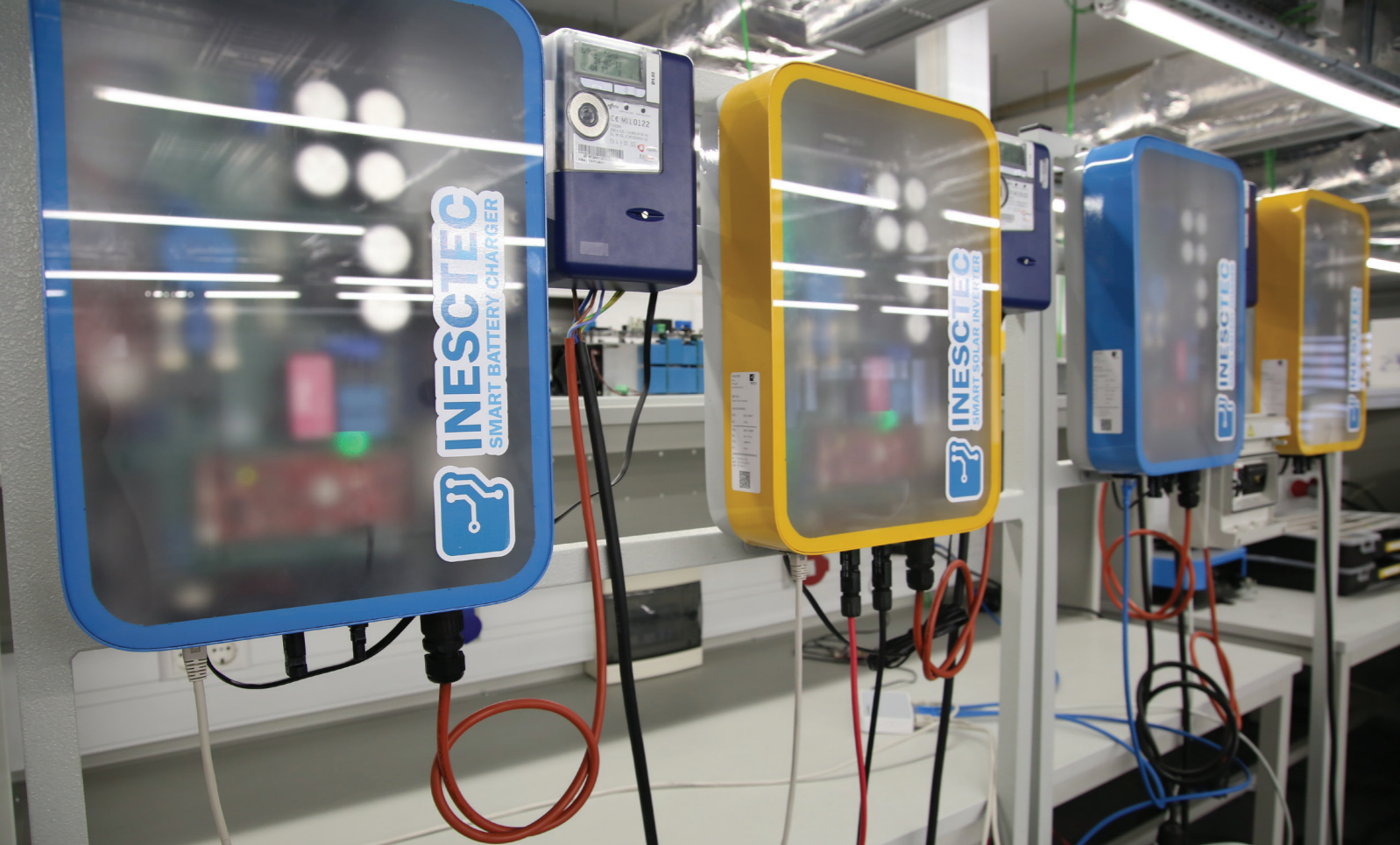
Figure 3 Smart energy inverters
